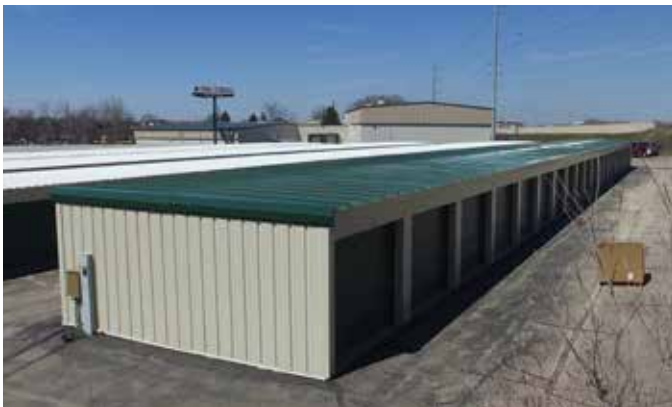
A freshly refurbished building with a new roof, reskinned walls, and new doors.
