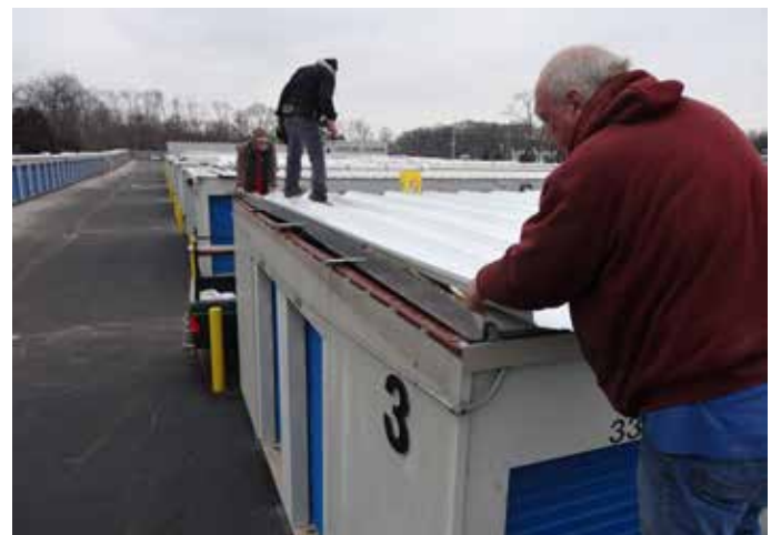
Finishing the reroof. New rake trim is added as part of the reroof process.
