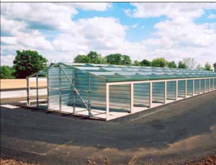
18. This endwall has no doors. The wall entire wall will be covered with A-panel.
