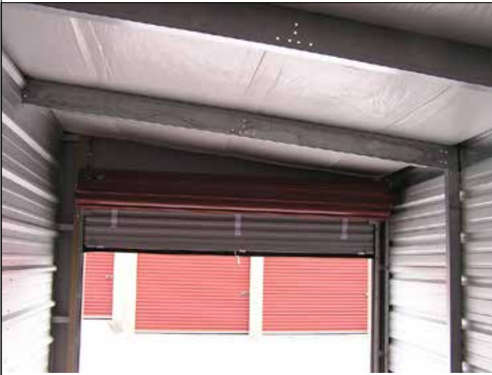
199. Here is a view of the inside of the unit looking out.
