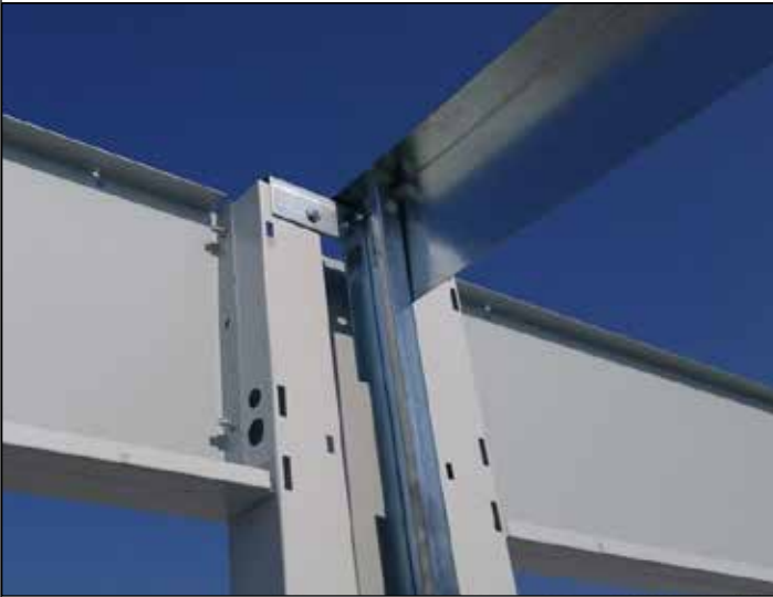
88. This is a photo of the field notched and installed rake angle at a sidewall jamb.
