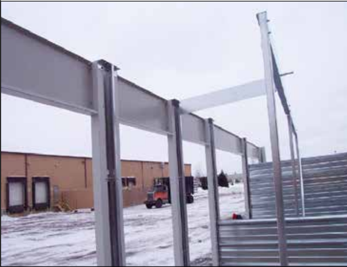
89. Field notch the rake angle. It is easiest to notch only one end. This photo shows the notched end at the purlin.
